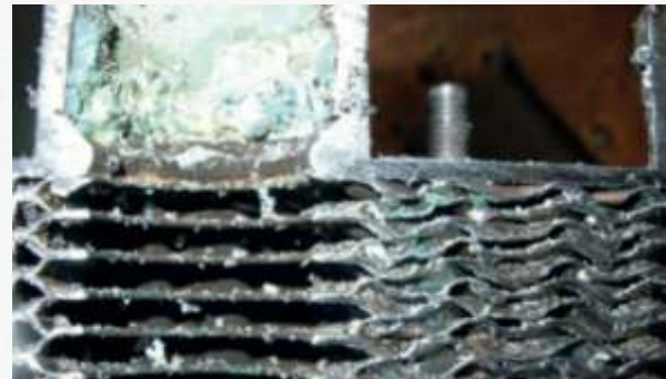
Figure 6: Limescaling in a heat exchanger
